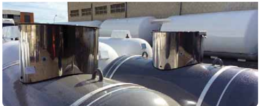
INSPECTION CHAMBERS ON UNDERGROUND TANKS
